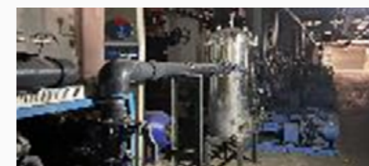
Xuzhou Xinyu Concentrated Water Recycling Unit
